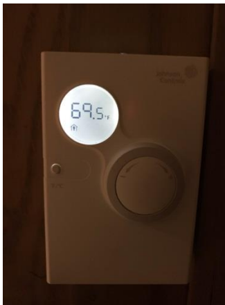
New "Smart" Thermostat in Each HS Classroom
